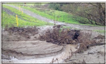
Fernandez Ranch. Collapsed culvert underneath the road blocks the channel with sediment.
