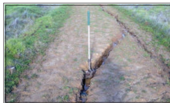
Sky Ranch. Ranch roads built 100 years ago lacked proper slope to provide for runoff.
